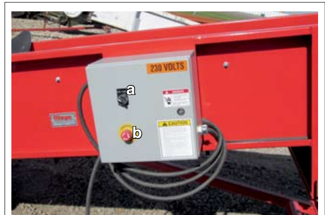
Control Panel (Typical)
